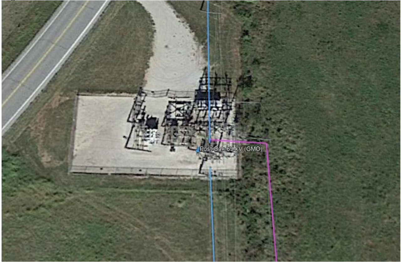
Figure 14 – Post Oak – 69kV Transformer
